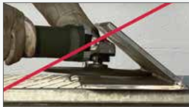
This solution violates safety standards
